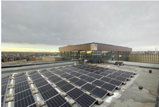
Solar panels – south roof
